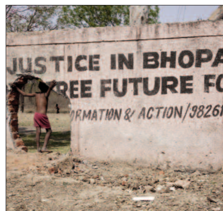
A boy standing by a hole in the wall surrounding the abandoned and derelict Union Carbide factory in Bhopal. Children play within the grounds despite the dangers from chemical contamination.
