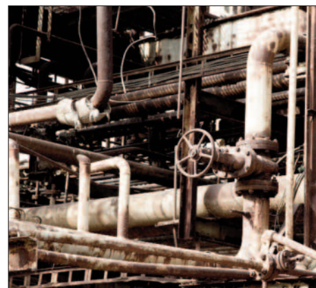
The faulty valve from the MIC plant in the abandoned Union Carbide factory.
